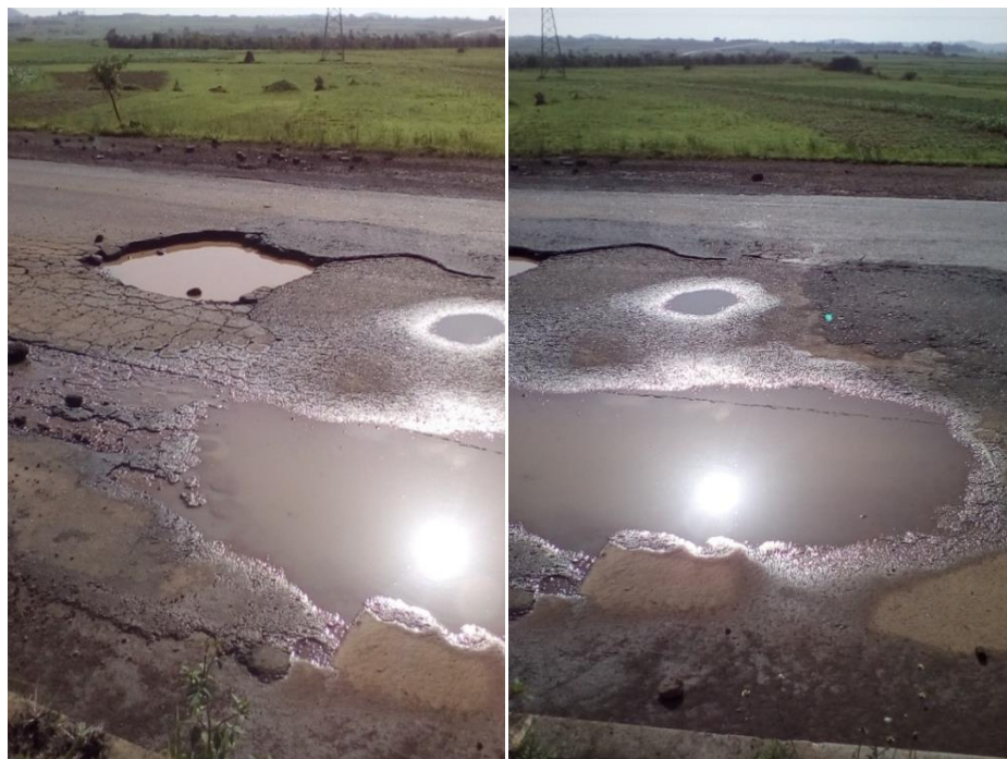
Plate 1: Failed segments of road at Bisichi Junction on the way to Mararaban Jama'a Plateau State.
