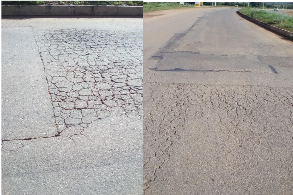
Plate 2: Failed segments of road at Kuru Jenta Junction Plateau State.
