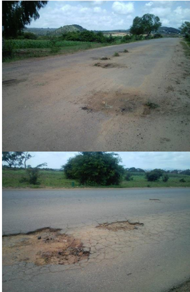
Plate 4: Failed segments of road at Dorowa, Plateau State.
