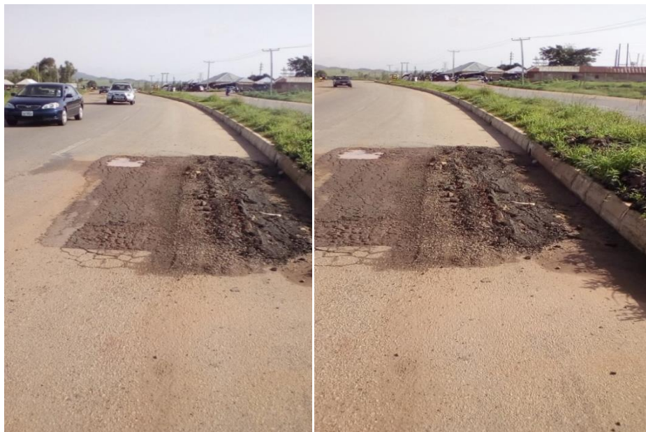
Plate 3: Failed segments of road just after Foron Junction enroute to the Polytechnic, Plateau State.
