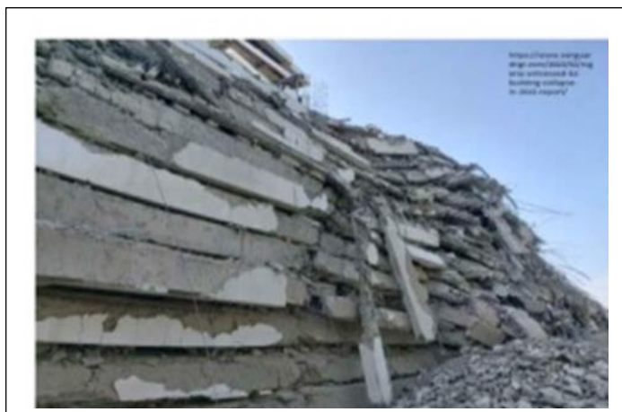
Figure 1a: Front View of Collapsed Structure (Source: Oke et al 2024)
