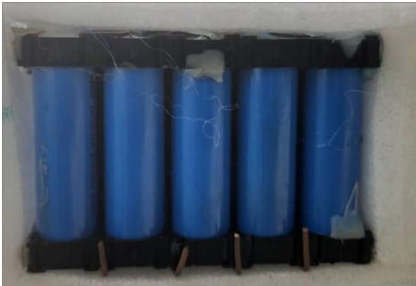
Figure 4c: Back view of 13.4 DC back-up from 18650 type of 46000 mAh Lithium-Ion Batteries Pack of 3.7 DC V (rechargeable) connected in series (S) and parallel (P).
