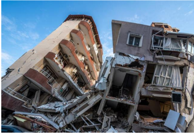
Figure 3c: Collapsed building after earthquake (Source: istockphoto, 2025b)
