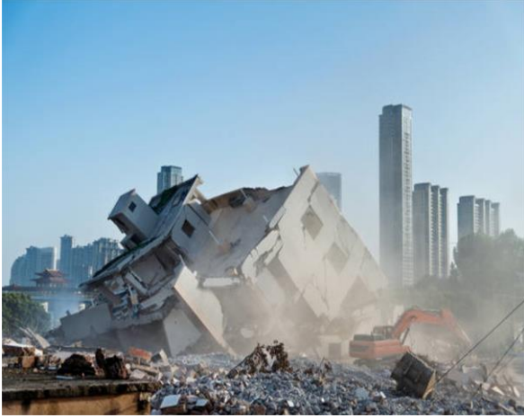
Figure 3b: Collapsed building during construction (Source: istockphoto, 2025a)
