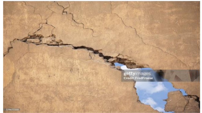
Figure 3d: Crack in the wall of a collapsed building after earthquake (Source: istockphoto, 2025c)
