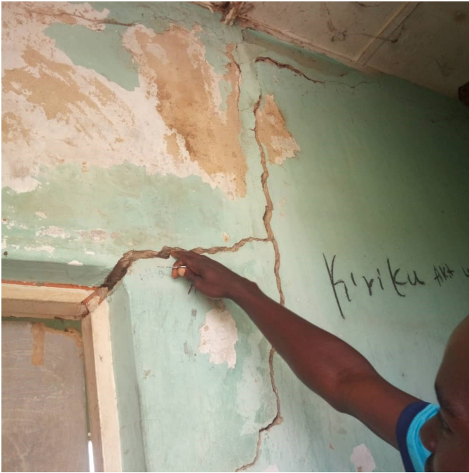
Figure 2. Observation of building cracks in the study area.
